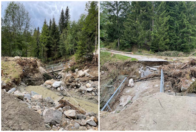
Fig. 1. Bridge after debris-flow impact, Carinthia, Austria 2022. (Image courtesy of Tazio C. Bernardi.)
