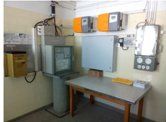
Figure 3: Grid-connection of new PV modules mounted at Jungfrauoch in 2014 (right), next to old ASP inverter from 1993 (left).
