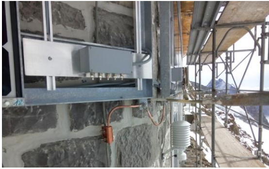
Figure 1: Installing new PV technology on the façade of the Jungfrauoch (3 454 m asl) research building in the Swiss Alps in autumn 2014.
