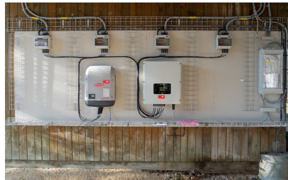
Figure 2b: Inverters and test surfaces at KNS test facility.
